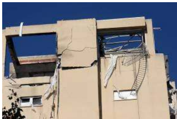
Apartment house in Ashdod takes a direct hit on January 1 (Roe I dan for the Sderot Media Center, January 1, 2009).
