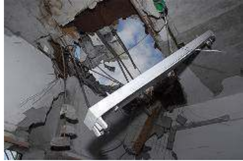
The hole ripped in the roof of a school classroom (Photo by Herzl Yosef, Ynet, December 30).
